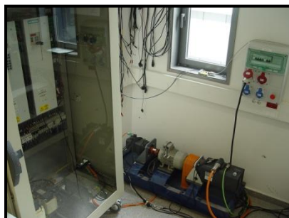
Motor Control Bench
